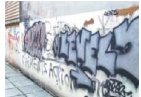
Inactive edges and poor maintenance of this area has resulted in this wall becoming increasingly problematic. If graffiti is not dealt with swiftly others will quickly add to it.
