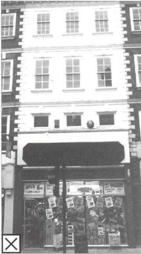
▲ A shopfront design that ignores the upper floors spoils the appearance of the building and the street scene
