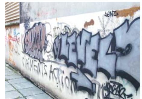
Inactive edges and poor maintenance of this area has resulted in this wall becoming increasingly problematic. If graffiti is not dealt with swiftly others will quickly add to it.
