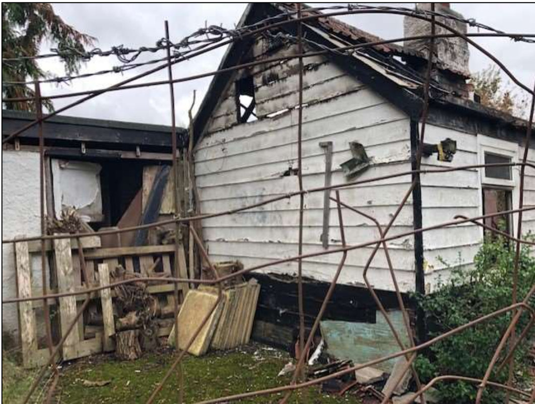
Plate 10: Oak Cottage, subject to recent fire damage.
