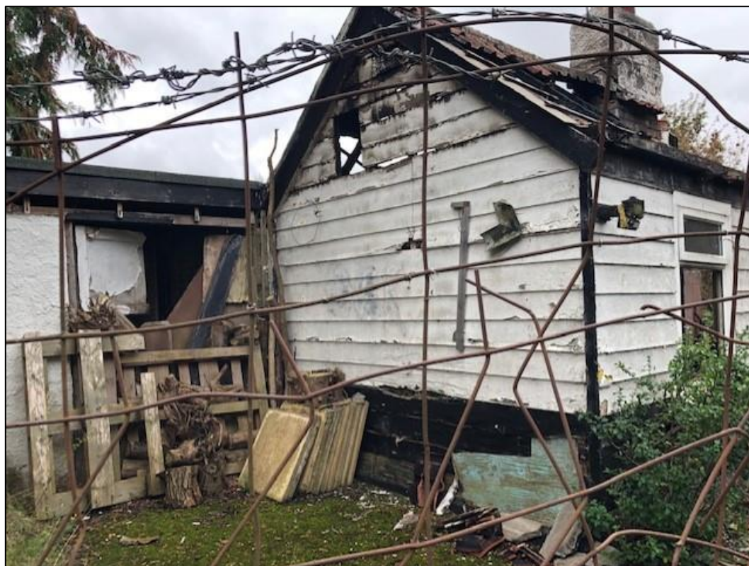
Plate 10: Oak Cottage, subject to recent fire damage.
