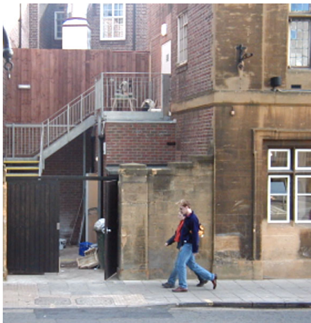
These gates have been used to conceal a bin storage area and provide security to an external staircase however they have not been properly managed or maintained and there is a limited sense of ownership. They are consequently left open creating an unattractive streetscape and compromising security.
