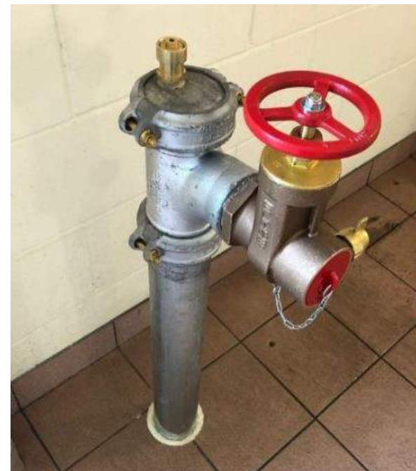
Exposed Landing Valve
