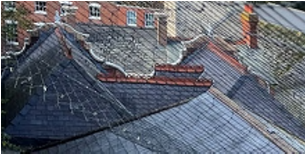
Photograph 2 - View looking towards Northgate Street showing the roof of the 1909/14 building as visible at the time of survey
