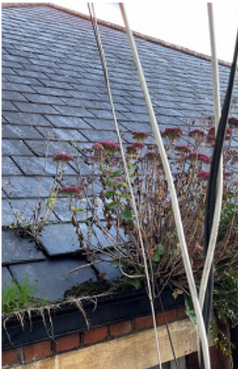
Photograph 9 – Lifted tiles on the Mezzanine building
