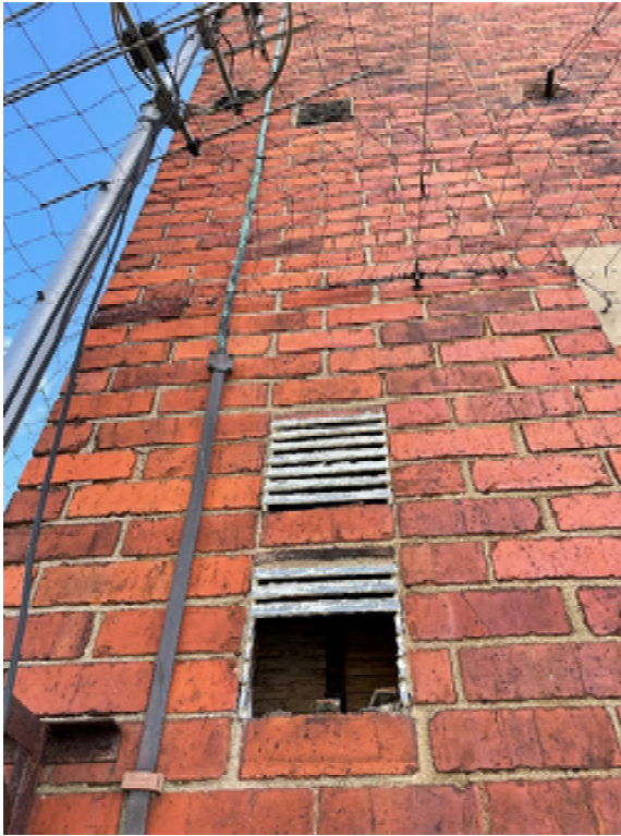
Photograph 7 – Example of broken vent on the Water Tower
