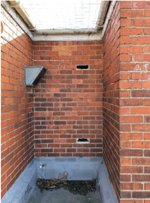
Photograph 5 – Missing bricks on Plantroom 1
