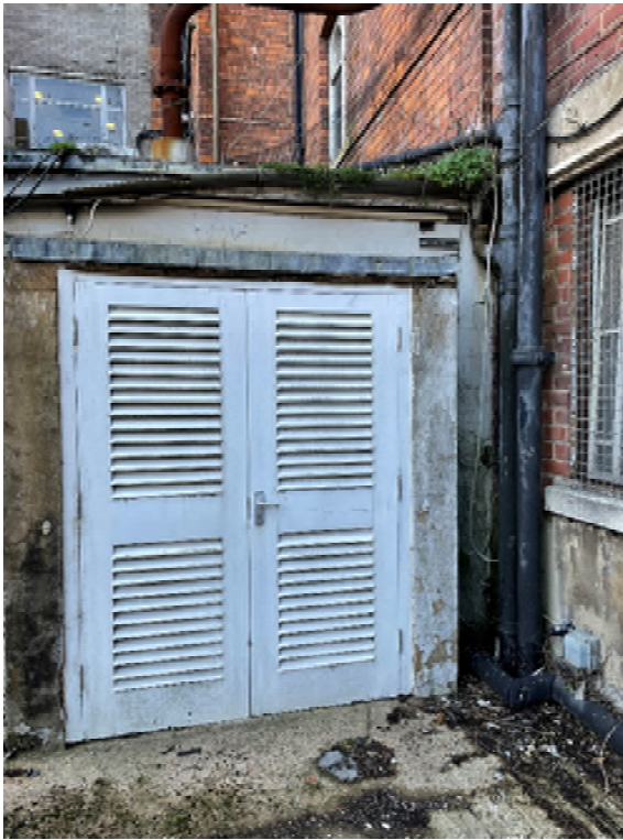
Photograph 11 – Gap in wall and lifted capping on the Generator building in the courtyard
