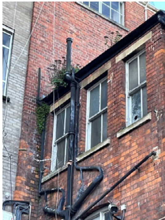
Photograph 10 – Broken windowpane leading into the Mezzanine building
