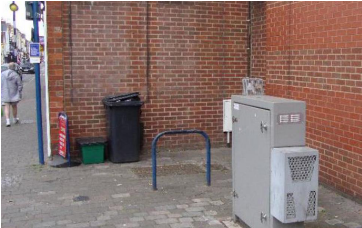
Figure 2-2 Photograph of Automatic Monitoring Site
