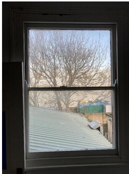
Figure 7 – Steel standing seam roof on rear extension (as viewed from first-floor window on rear elevation)
