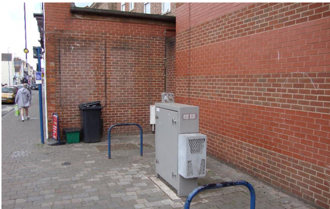
Figure 2.1 Teledyne chemiluminescence Nitrogen Oxides Analyser in Barton Street
