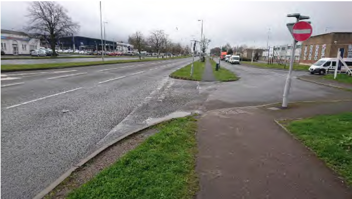
Figure 2: Evidence of kerb overrun.
